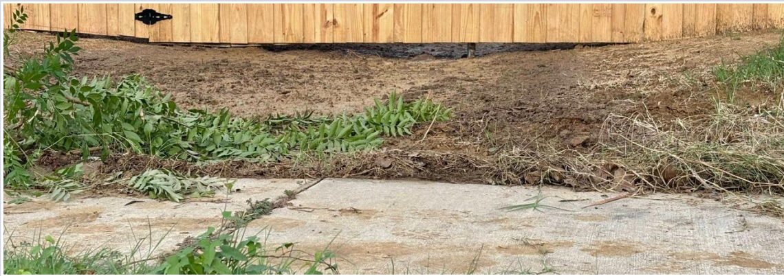
Runoff 5 — low opening and wet/eroded path beneath the fence.
