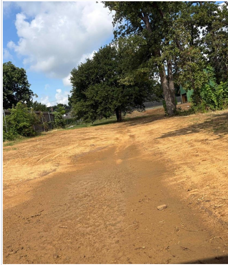
Runoff 2 — wet flow path visible along compacted/exposed soil.
